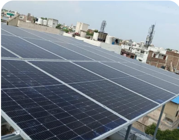
850KWP SOLAR INSTALLATION AT SOUTHEAST LTD. SREL
