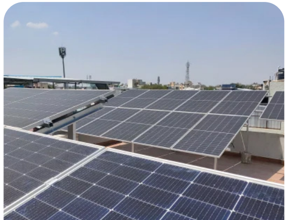
1200KWP SOLAR INSTALLATION AT OFMA LTD. KEPZ CHITTAGONG UCC.
