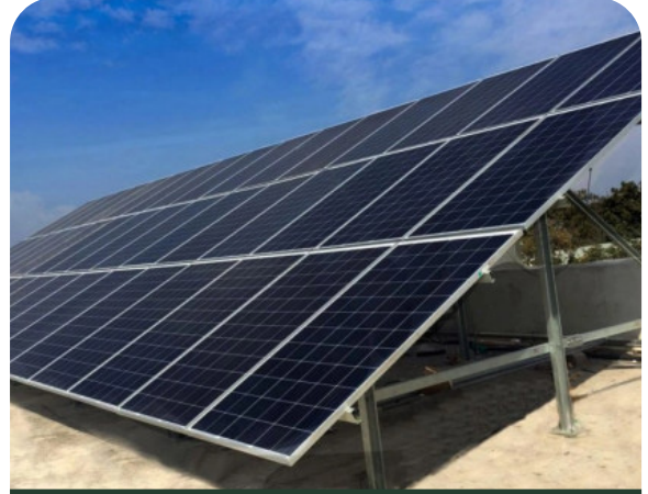
128KWP SOLAR INSTALLATION AT SF FASHION, DANA POWER CO. LTD.
